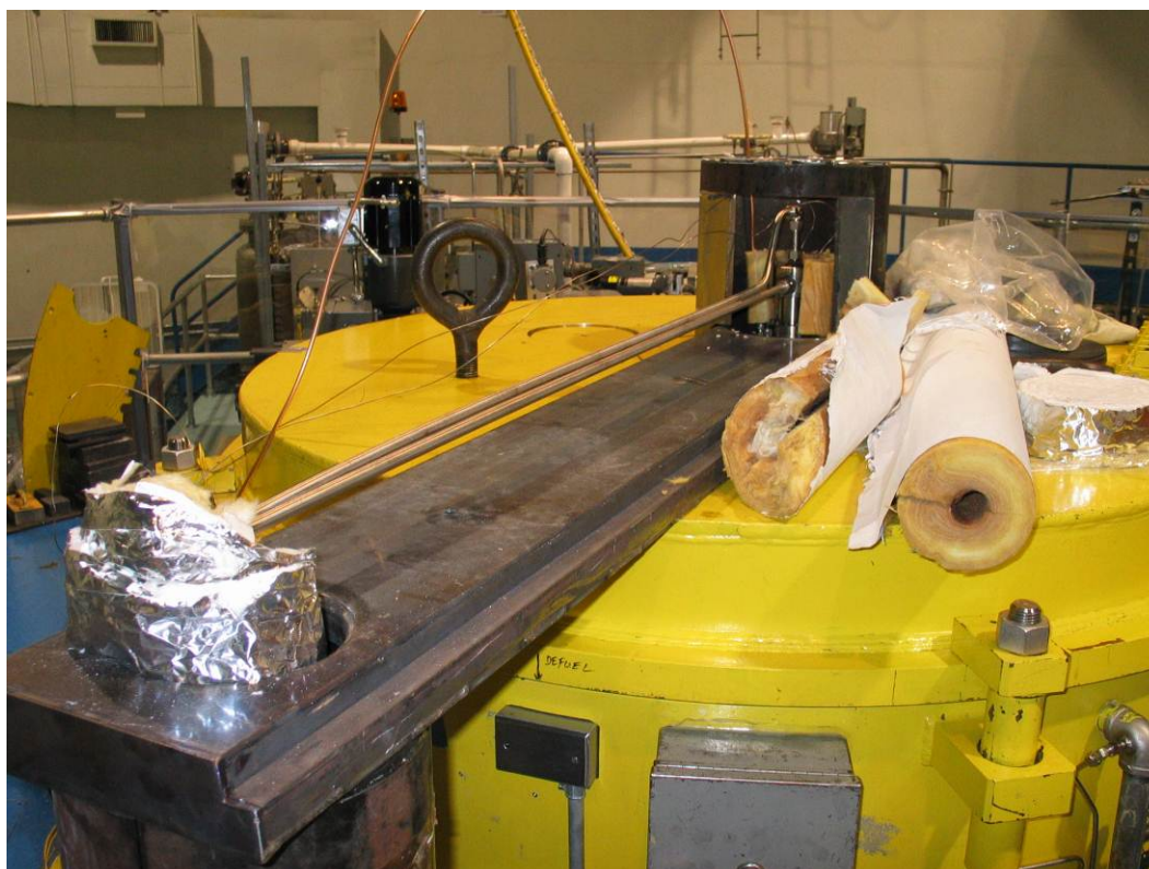
Figure A4. The ACI top head and coolant lines after facility installation in the MITR and during installation of the thermal insulation and shielding.
